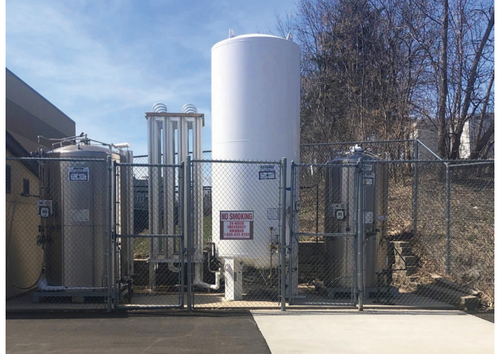
Super Radiator Coils' micro-bulk storage tanks
